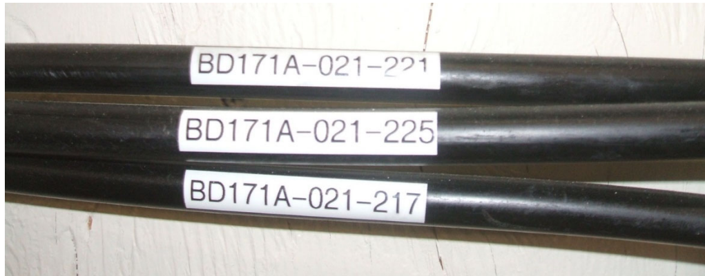
Figure 102: Hard-line CATV Cable label between MDF and MDF (Building 171A-Room 21 to Building 171A-Room 217).
