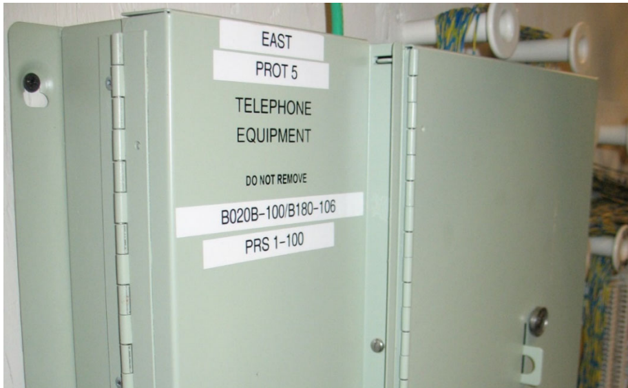
Figure 106: Protector labeling for a cable pairs 1 through 100 that goes from building 20B, room 100 (only room in building) to building 180, room 106.
