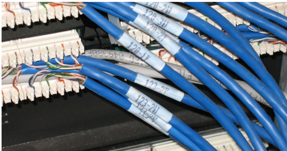
Figure 107: Structured Cable, CAT 6, labeled with the faceplate room and port served.
