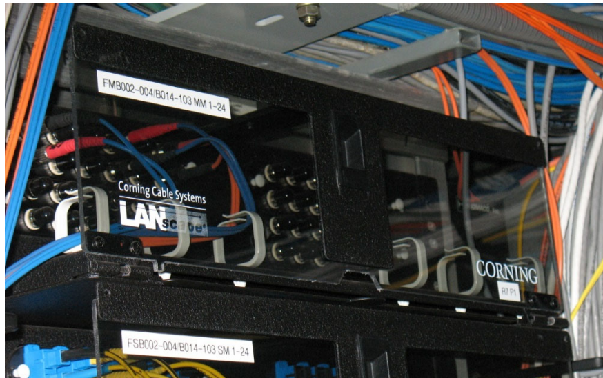
Figure 103: Labeling of a fiber shelf in a rack (Fiber- Multimode-Building 2 to Building 14-Room 103- Multimode strands 1 to 24).
