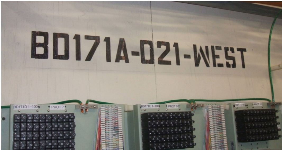
Figure 101: Backboard label to be stenciled on appropriate MDF/IDF/SCF wall (Building 171A, Room 21 – West Wall) in every telecom space.
