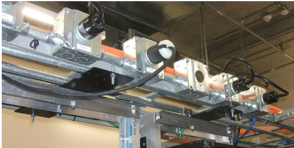
Exhibit 11 - Electrical Over Racks
