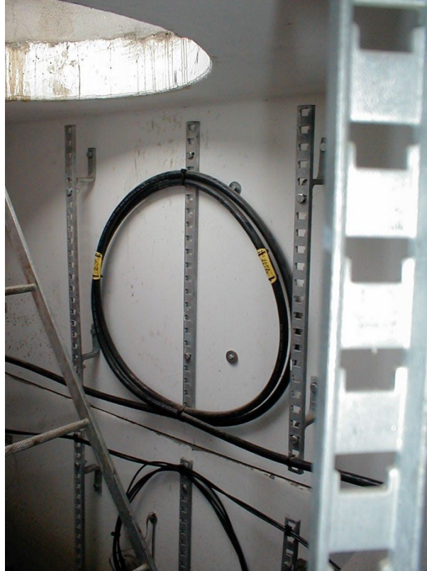
Exhibit 1 - Fiber Service Loop in a Manhole
