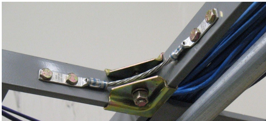
Exhibit 13 - Cable Tray Grounding
