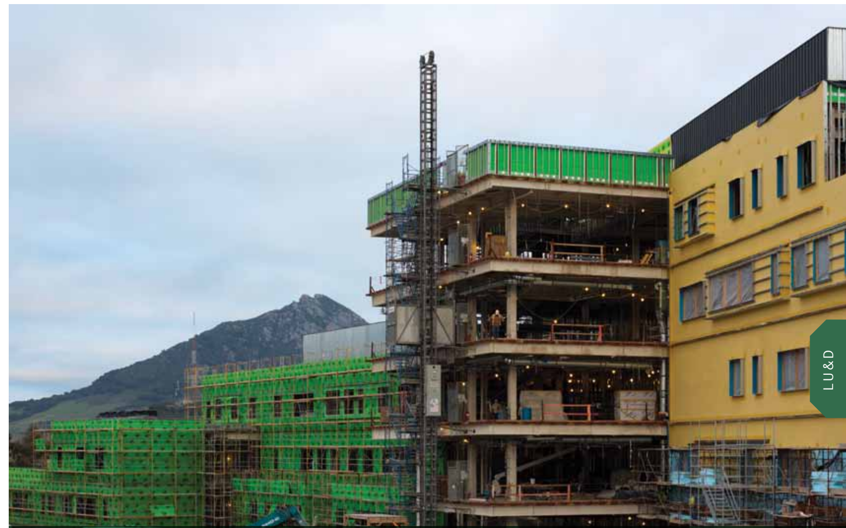
The Center for Science and Mathematics replaces a one-story building that was more than 50 years old. The new building not only provides better research and educational facilities, but also more efficiently uses valuable land in the campus core and has been designed with modern water and energy conserving features.
