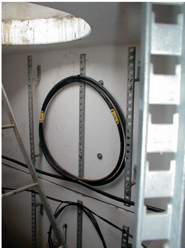
Exhibit 1 - Fiber Service Loop in a Manhole
