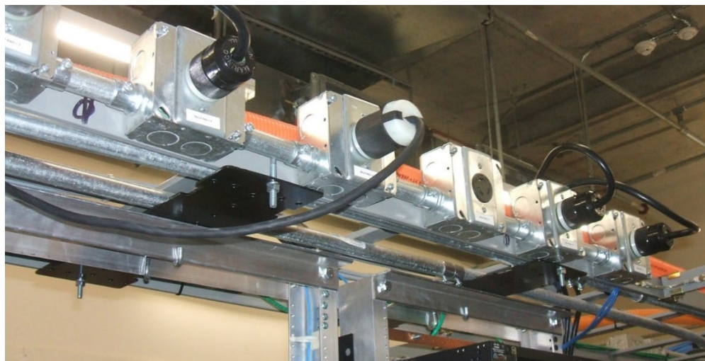
Exhibit 11 - Electrical Over Racks
